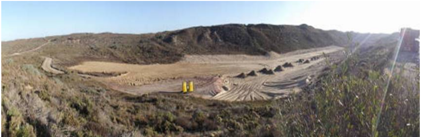
M4 Remediation Site; placing vegetative overburden on post excavation site. Note: filled wetland located on right-hand side of project site (area with slightly darker sand).
