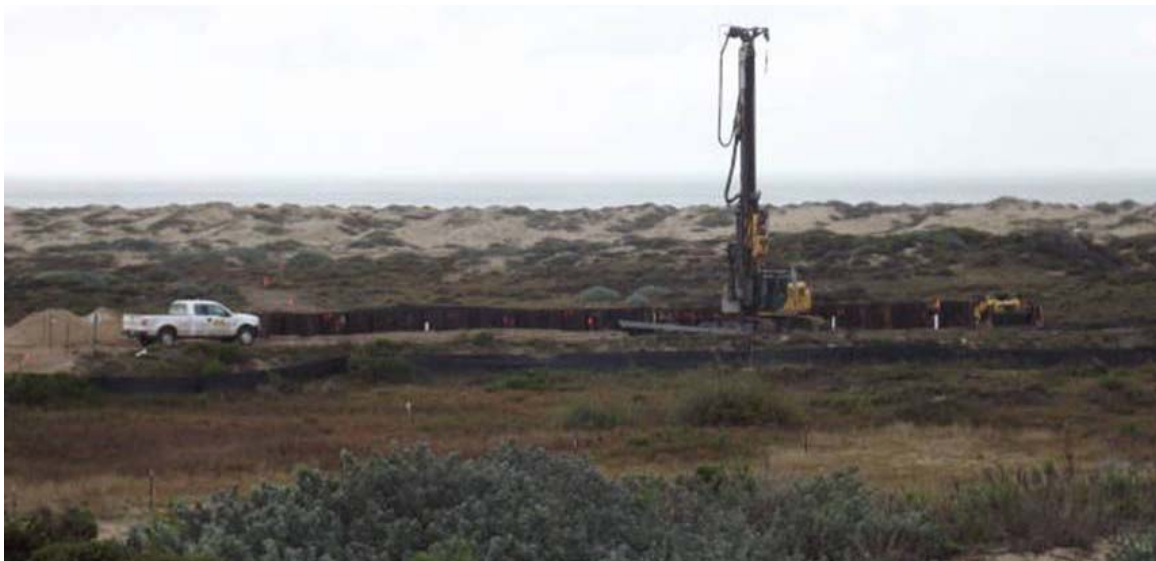
B2 Installing sheetpile around the final cell of contaminated material at this site.
