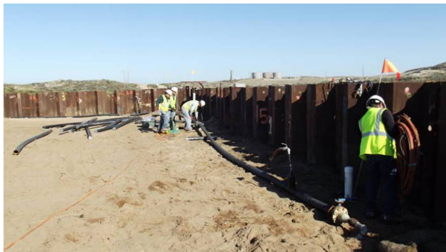
B2 Site: installing piping for the dewatering system inside the sheetpile wall.
