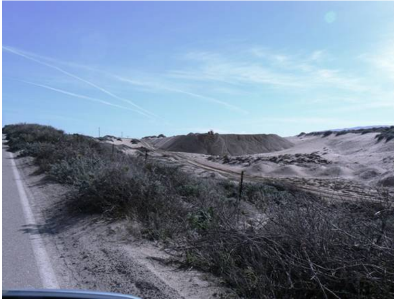
E4A clean overburden stockpile site (site now contains at least 37,125 cubic yards of clean overburden from the B5A site).
