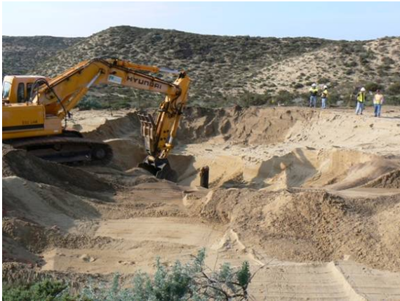
F11 pad and access road removal. Diluent-contaminated soils were exposed (more than 8 feet deep) during the removal of the redrock and base material on the pad site. Chevron is currently “chasing” contamination and coordinating with the RWQCB.
