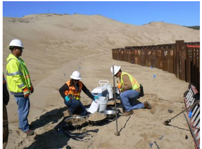
B5A: collecting hand augers outside the sheetpile wall to characterize extent of contamination south of remediation site.
