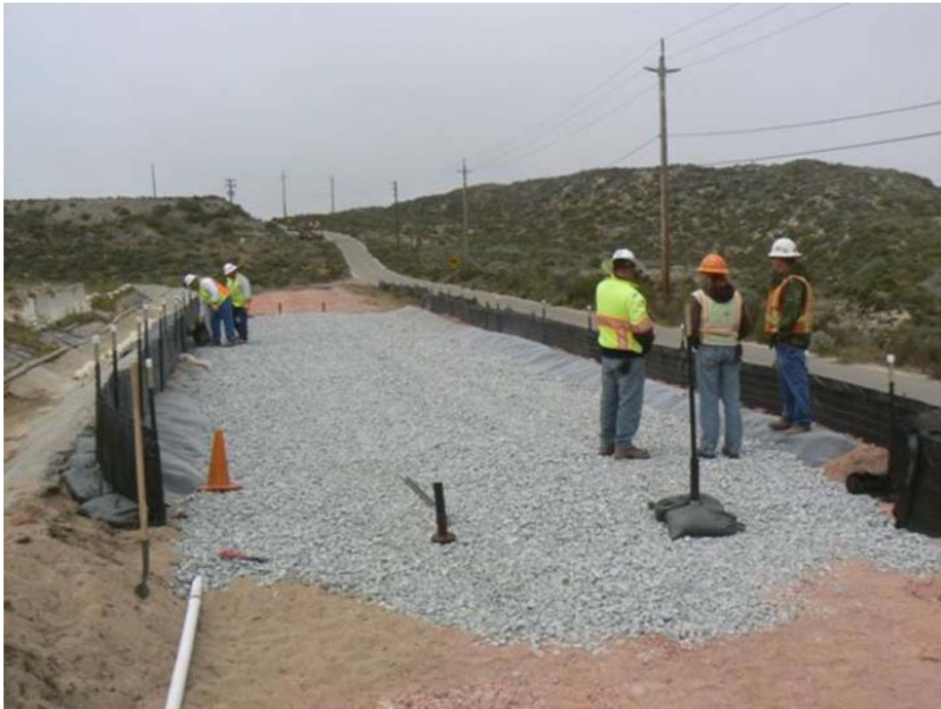
Building a new and improved Decontamination Pad outside the TB9 Stockpile Site.
