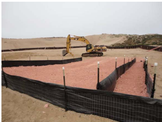
Building a new and improved Decontamination Pad within the B5A Excavation Site.
