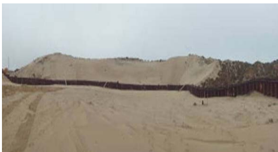
View of dune to the immediate south of B5A Site (location of dirty material that will be excavated outside the B5A Sheetpile wall).
