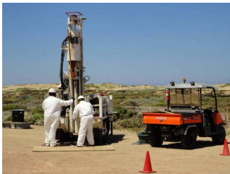
Bore samples being collected at the B2A Excavation site to better characterize extent of contamination and to also collect needed archaeological information at a suspected cultural site.
